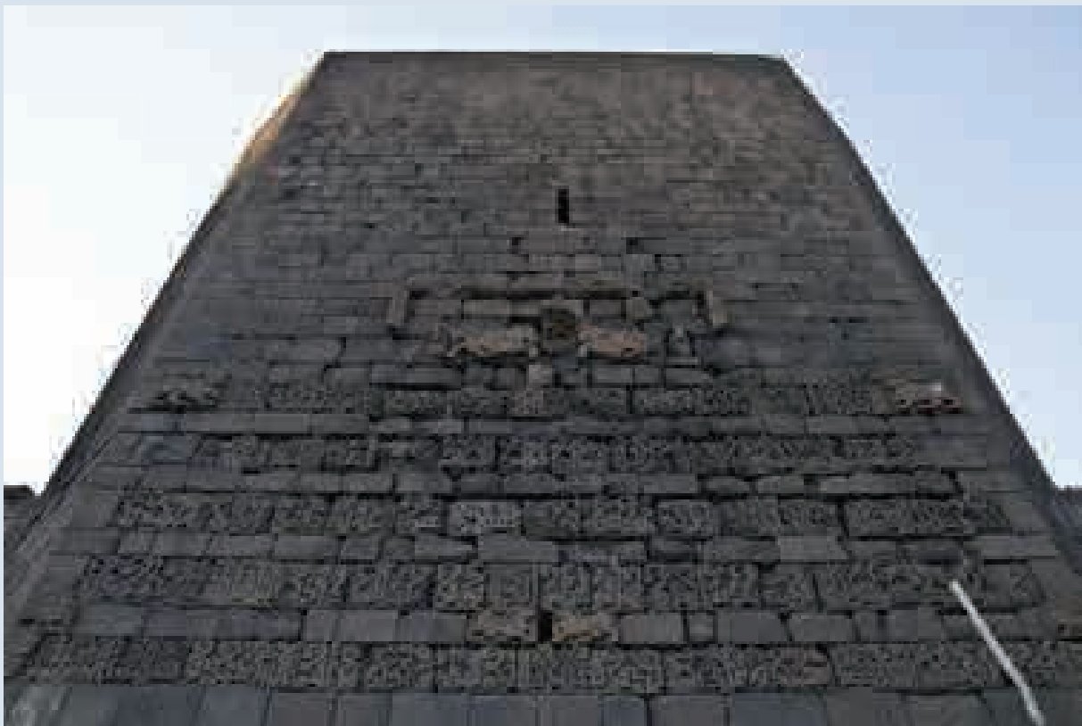
Melikşah / Nur (Melik Shah / Light) Tower (Merthan Anık, Diyarbakır Metropolitan Municipality Archive)
